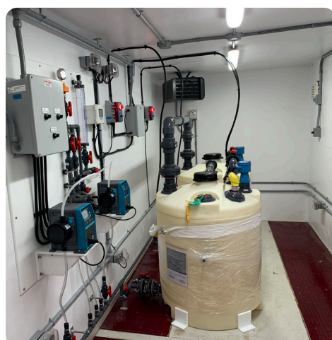
De-chlorination container for a wastewater treatment plant. Designed with room for future system expansion.
